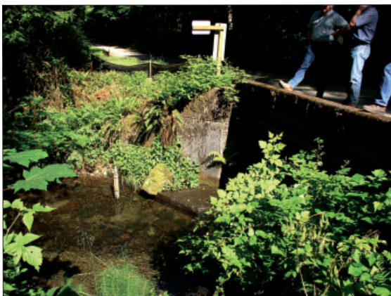
A turbidity sensor was installed in a tributary of the Cedar River watershed to monitor water quality conditions for the city of Seattle, Washington.
